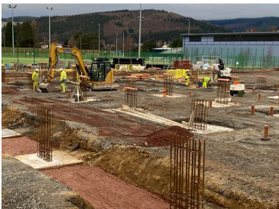
Preparation for the ground floor slab, including drainage pop-ups, pad foundations and column starters
